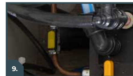
GAS ISOLATION VALVE
