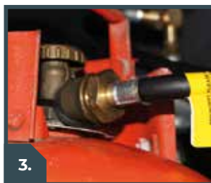
GAS HOSE CONNECTION
