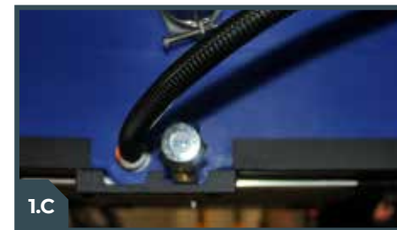
1.C WATER TANK TAP
