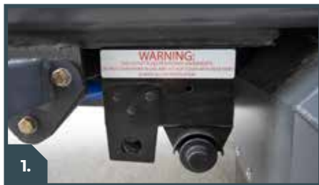
1. GAS OUTLET FLUE
