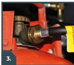
GAS HOSE CONNECTION
