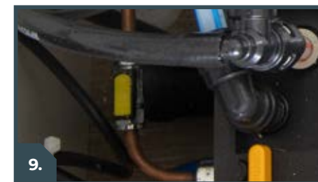
GAS ISOLATION VALVE
