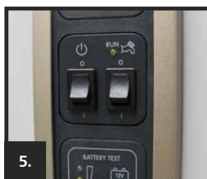
5. MAIN & RUN SWITCH ON
