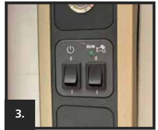
3. CONTROL PANEL ON
