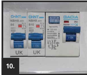
10. LOCATION OF CIRCUIT BREAKERS
