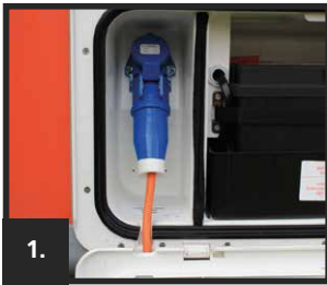
1. POWER SUPPLY TO OPUS
