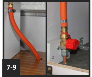
7-9 GAS FITTING / VALVE
