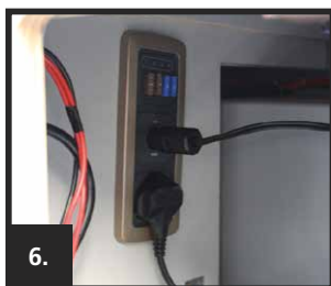
6. FUSE BOX LOCATION
