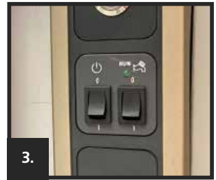
3. CONTROL PANEL ON
