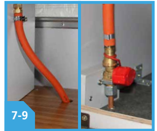
7-9 GAS FITTING / VALVE
