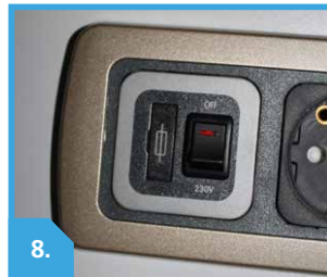
8. SWITCH OFF HEATER ISOLATION SWITCH
