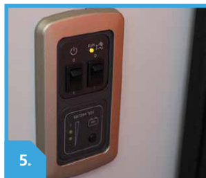
5. MAIN & RUN SWITCH ON
